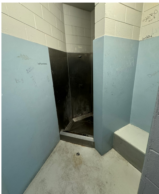
Photo 15 - Shower in the Women's and girls' unit at the Cairns watch-house, as seen from the doorway.
